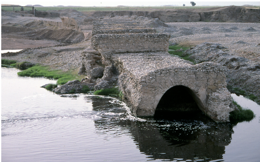
Figure 11. View of the inverted siphon and the piers of the overlying bridge at Jundi Shapur (photograph: author, 2003)
