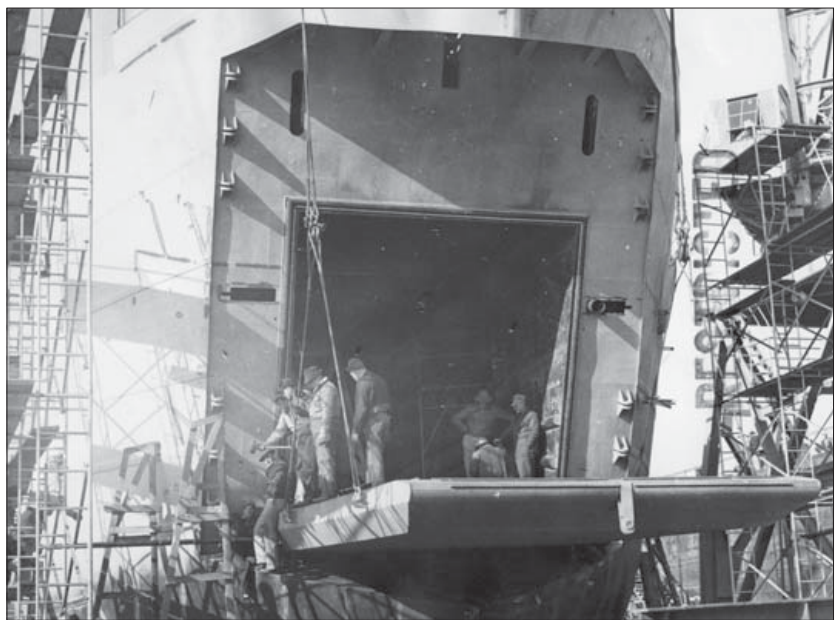
LST-157 under construction at Evansville, Indiana. Temporary cables support the ramp. The horizontal slots are for the geared door-closing ratchet and the upper vertical slots for the ramp chains. The heavy-duty door hinges can be seen along the sides. (Collection of the Evansville Museum of Arts, History and Science)
