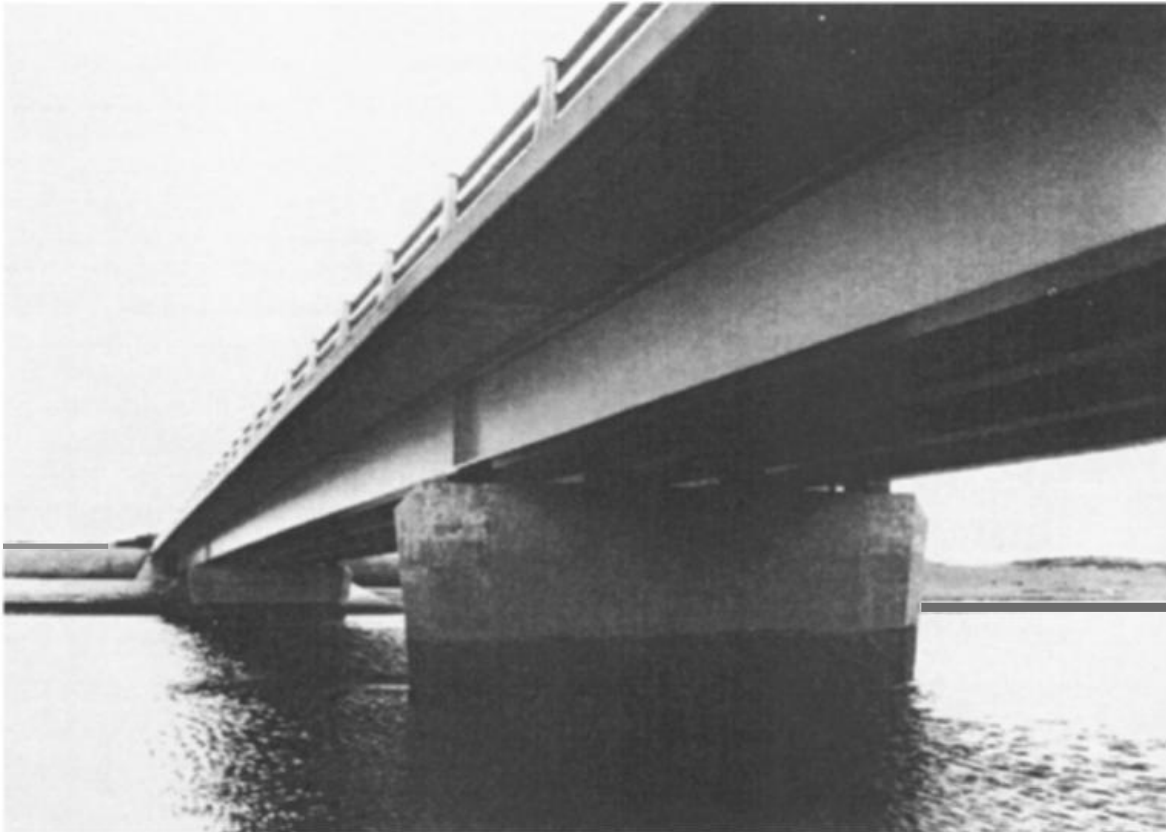
Fig. 1.10 Steel composite beam-and-slab bridge at Newburgh, Scotland; designed by Grampian Regional Council. Photograph courtesy Grampian Regional Council.
