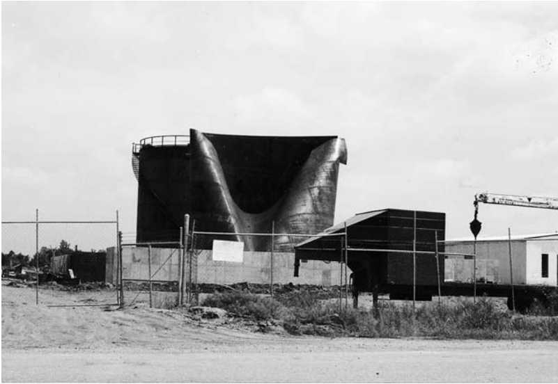
Plate 2.2 Relatively moderate wind caused collapse of tank during construction due to insufficient bracing.
