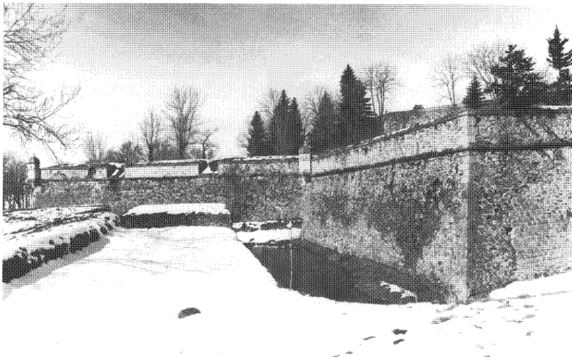
6 View down a covered way to a snow-topped traverse (Mont-Louis). The covered way is commanded by a ravelin (right), and by the embrasures of the bastion face beyond
