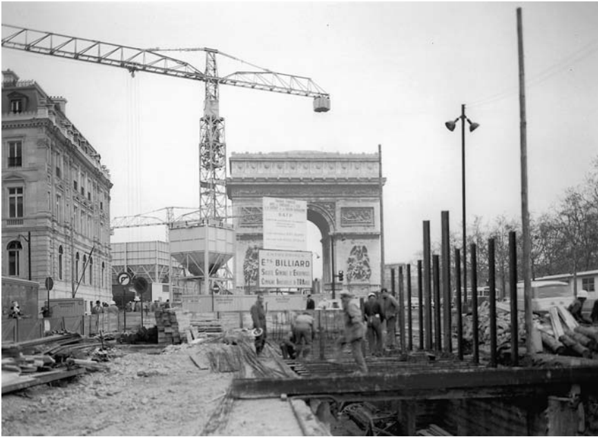
Figure 0.1 The Arc de Triomphe surrounded by cranes during construction of the RER station beneath place de l'Étoile, January 1964.
