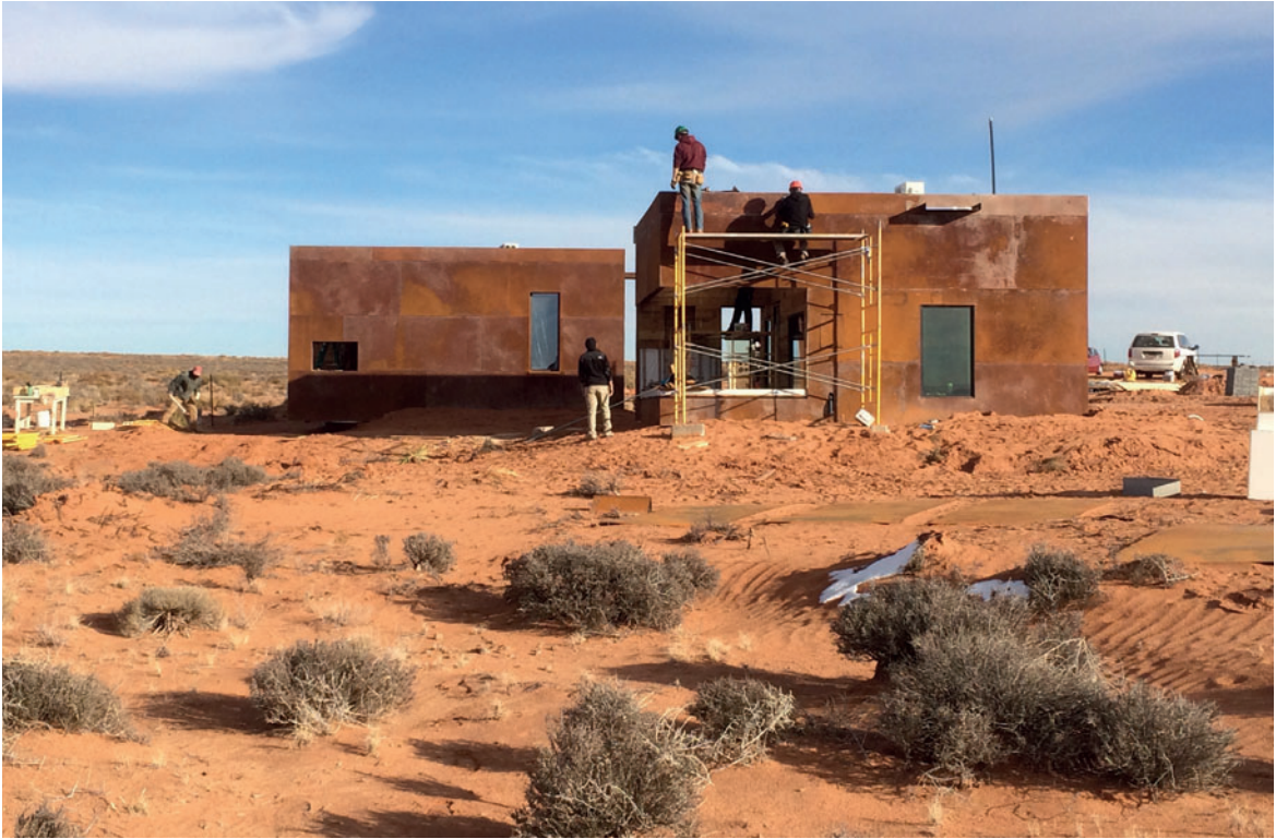
Figure 0.6 Building the Mexican Water Cabins, DesignBuildBLUFF, Mexican Water Cabins, Navajo Nation, Utah, USA, 2014
