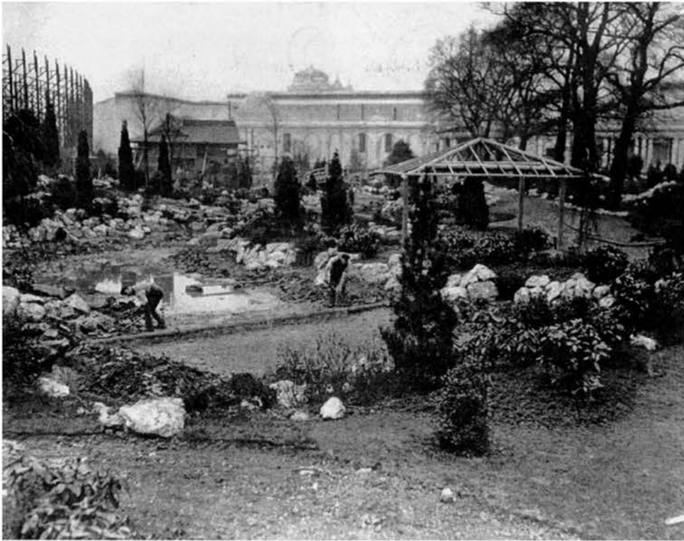
Figure 7. "Garden of Peace" under construction at the Japan-British Exhibition. Source: Private Collection
