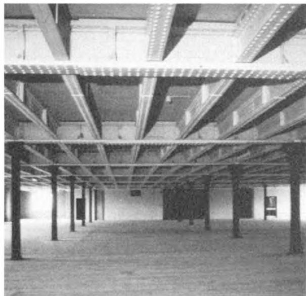
Fig. 9 Fairbairn-type wrought iron frame LNWR warehouse, Manchester, 1869 interior after conversion (engineers LNWR company).
