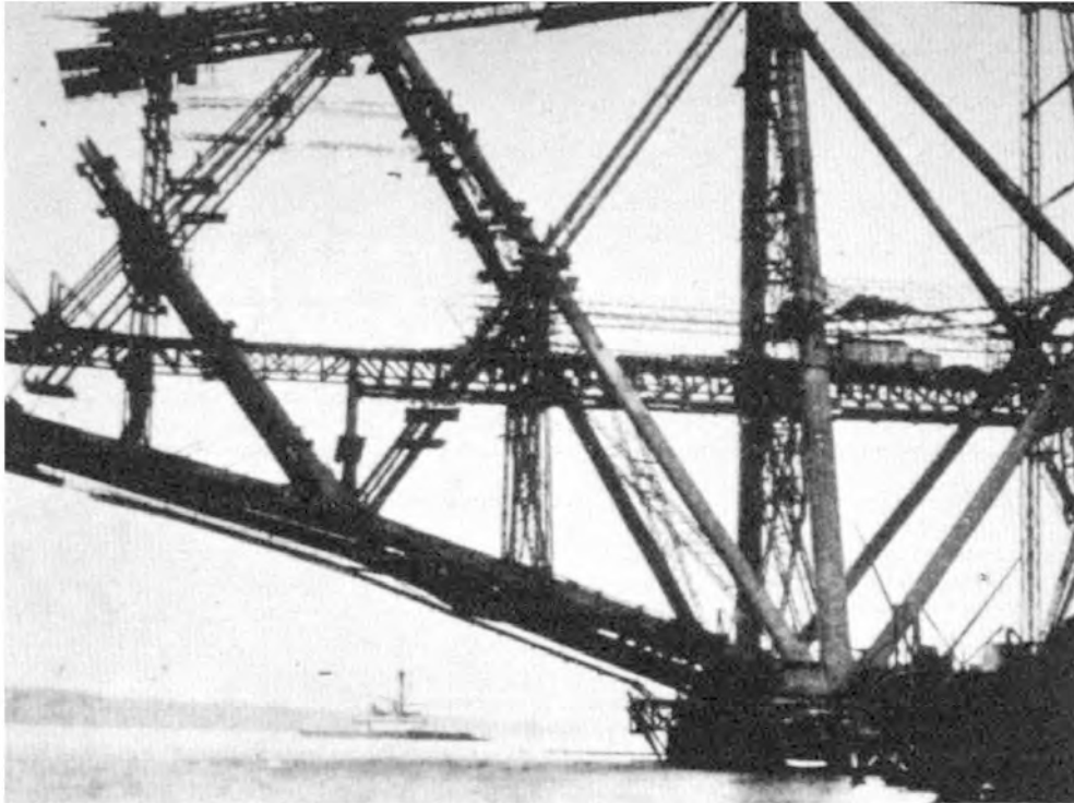
Fig. 21 Construction of cantilevers to the Firth of Forth railway bridge (refer also to lead-in picture to chapter 7).
