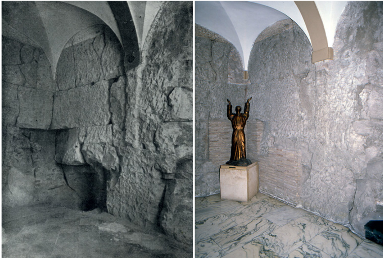
Fig. 33 The recess for the corner truss in the 1940s and after the restoration of the wall, inside the Monastery of SS. Cosma e Damiano (left: from Castagnoli, Cozza 1956–1958, fig. 14; right: photo author; cfr. Fig. 126).
