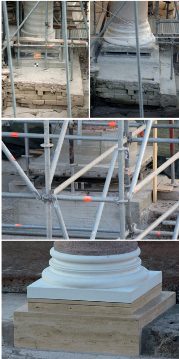
Fig. 17 Top: base of the first column (toward the Basilica of SS. Cosma e Damiano) being constructed (photos author). Center and bottom: base of column A “inaugurated” on April 21, 2015, and at the end of the reconstruction (photos Massimiliano Forconi).
