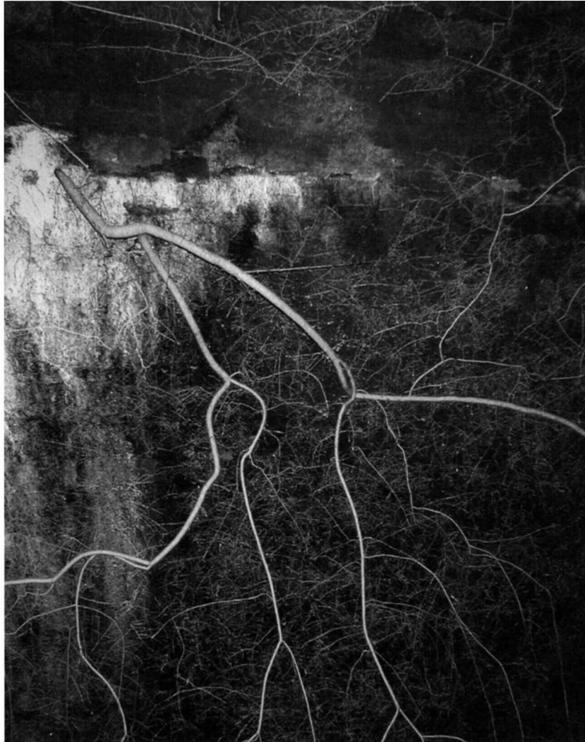
Figure 2.1 Roots inside the long-abandoned Croton Aqueduct in the Bronx
