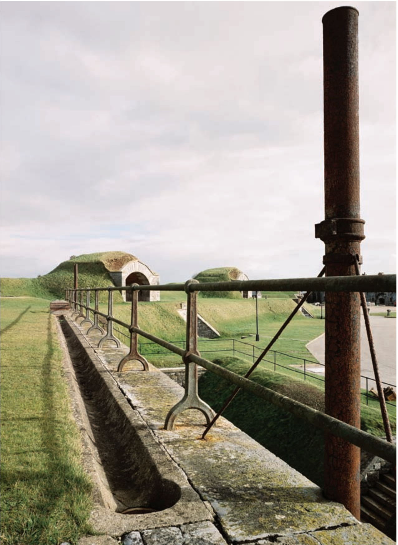
Plate 8 Fort Tregantle. Northern ramparts with Haxo casemates, handrail and gutter. (© English Heritage. NMR, AA000724)
